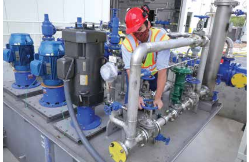
In 2020, SwRI completed construction of the STEP sCO 2 pilot plant building. We are now installing reconfigurable skid-mounted components, which allows the facility to evolve and keep pace with advancing technology.
