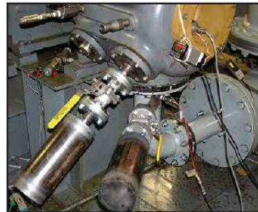
■ Figure 25. Prototype VOs installed at the cylinder nozzle and valve cap.
