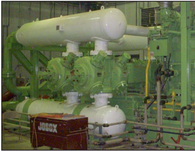
Figure 5: Field site for pulsation and performance testing of DDV cylinder.
