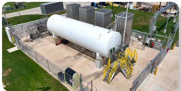
SwRI's liquid hydrogen tank facility holds a nominal 4,000 kg (17,500 net gallons) and can deliver 150 kg/hr at 350 bar.
