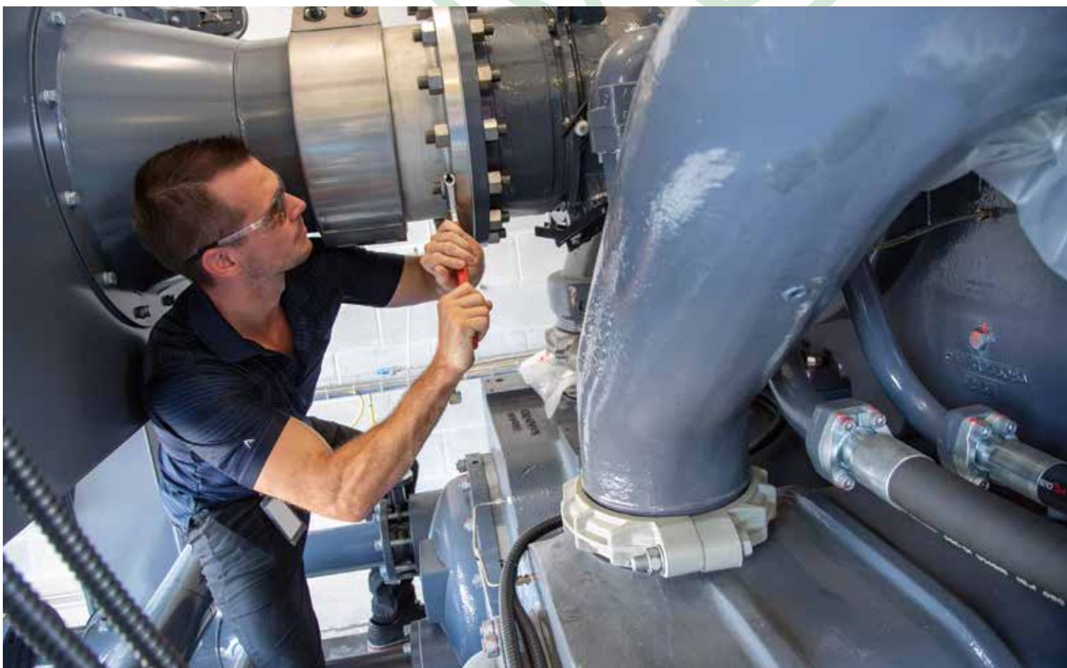
SwRI's High Energy Annex Test (HEAT) combustion facility includes a new, powerful air compressor to explore how alternative fuels affect the performance of gas turbine combustion systems.
