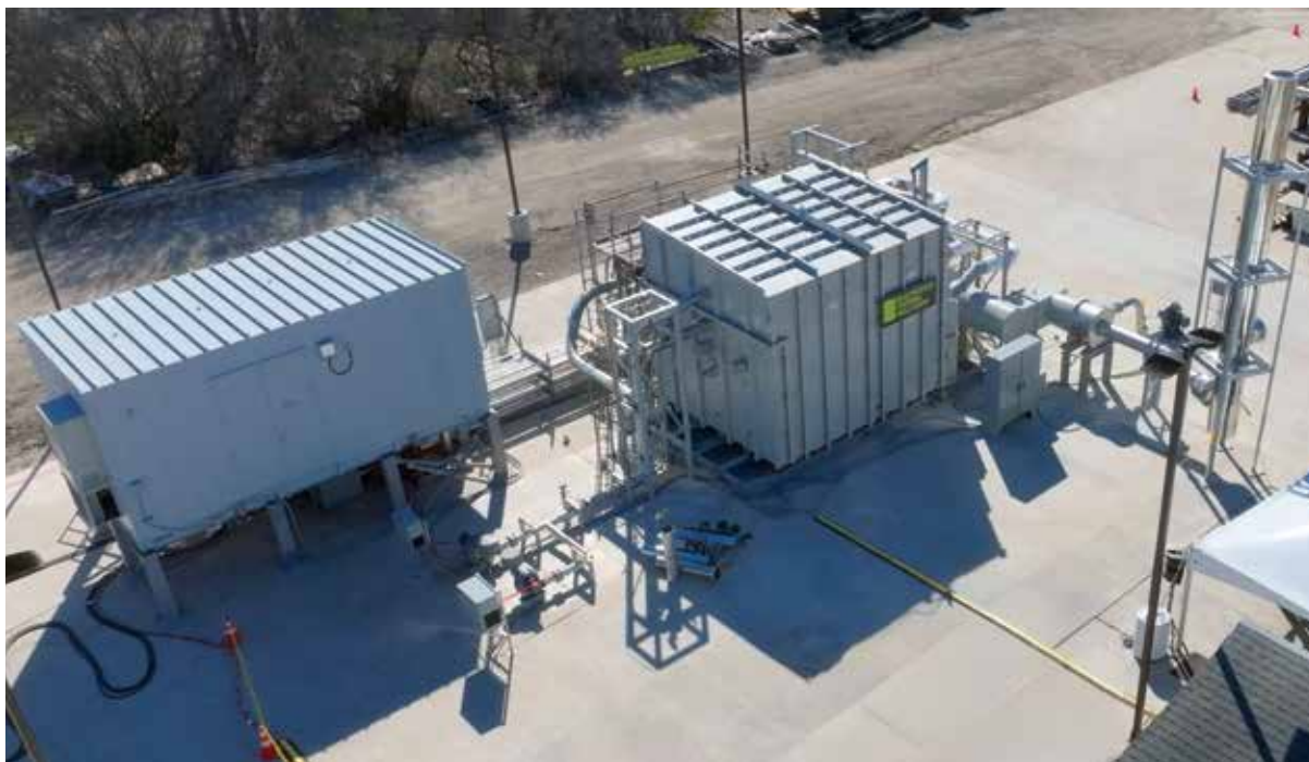
SwRI is testing a client's 20 MWh, 1,800 degrees Celsius thermal storage system at its upgraded HITECS site.
