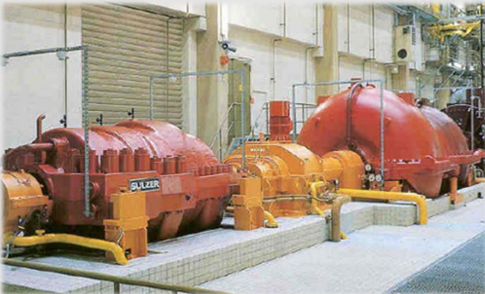
Huntorf Charging Compressor Train
