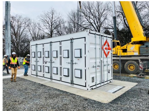
EnerVenue at McAlpine Creek Substation
