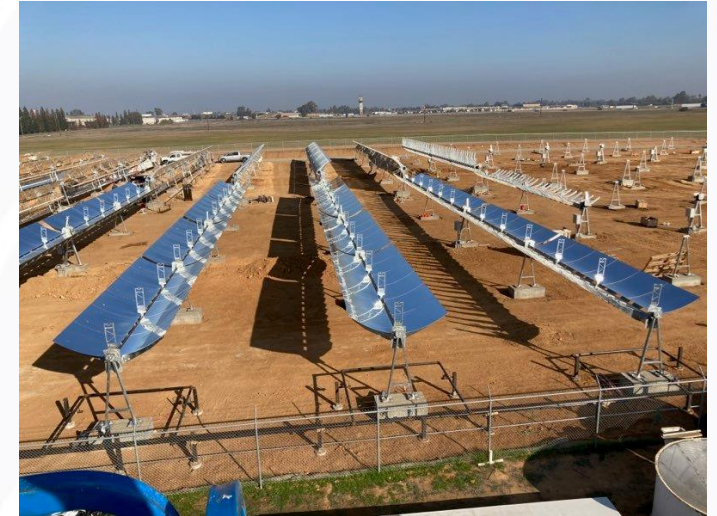
SunVapor's Two Solar Industrial Process heat facilities for Dimethyl Ether Production & Almond Processing
