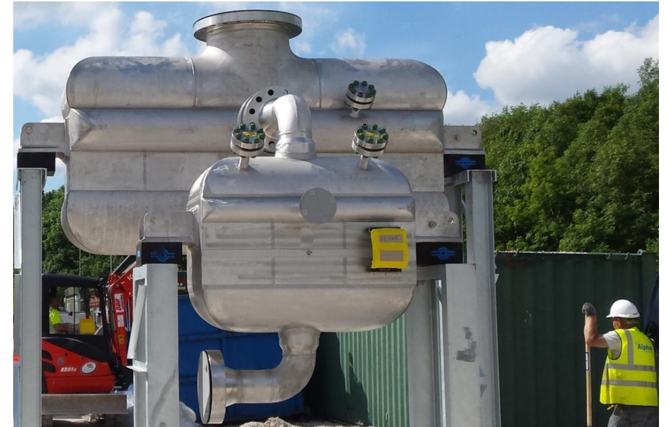
Bury Demo site Evaporator and HX1 (front)
